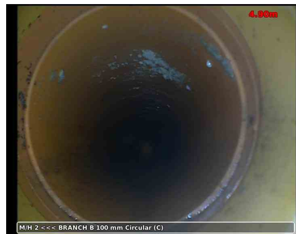
20211118-122550-snap0003.jpg, 00:01:00, 4.90 m Pipe material changes to polyvinyl chloride at this point
