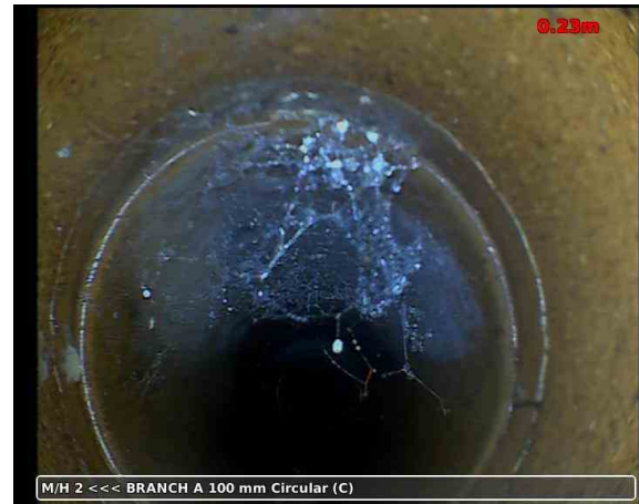
20211118-122214-snap0001.jpg, 00:00:12, 0.19 m Crack, circumferential from 12 o'clock to 12 o'clock
