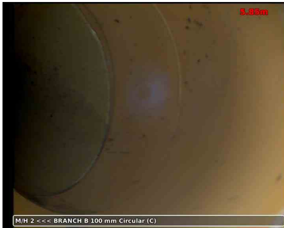
20211118-122550-snap0004.jpg, 00:01:09, 5.85 m Line deviates left
