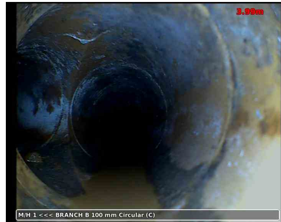
20211118-111716-snap0001.jpg, 00:00:30, 3.99 m Junction at 9 o'clock, 100mm dia
