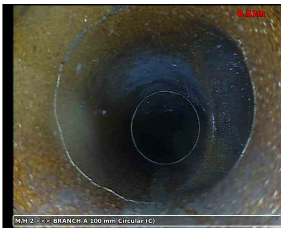
20211118-122214-snap0002.jpg, 00:00:24, 0.57 m Crack, circumferential at joint from 12 o'clock to 12 o'clock
