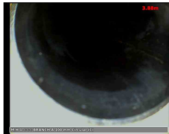
20211118-111324-snap0003.jpg, 00:01:02, 3.88 m Finish node, rodding eye, reference: BRANCH A - INTERNAL STACK
