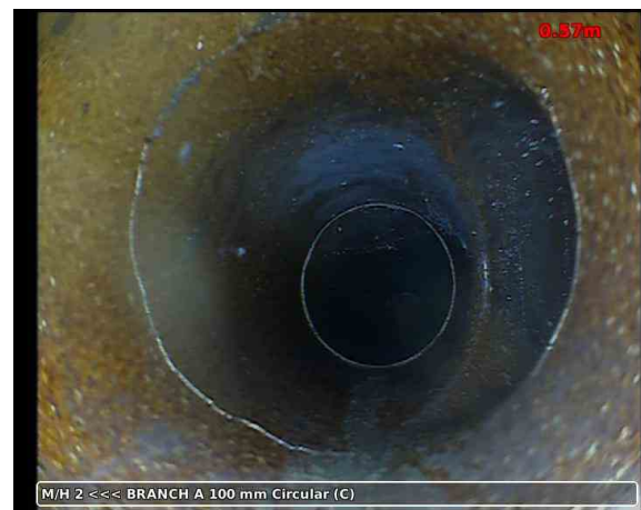
20211118-122214-snap0003.jpg, 00:00:34, 0.57 m Junction at 3 o'clock, 100mm dia
