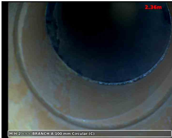
20211118-122214-snap0004.jpg, 00:01:40, 2.36 m Finish node, rodding eye, reference: BRANCH A - INTERNAL STACK
