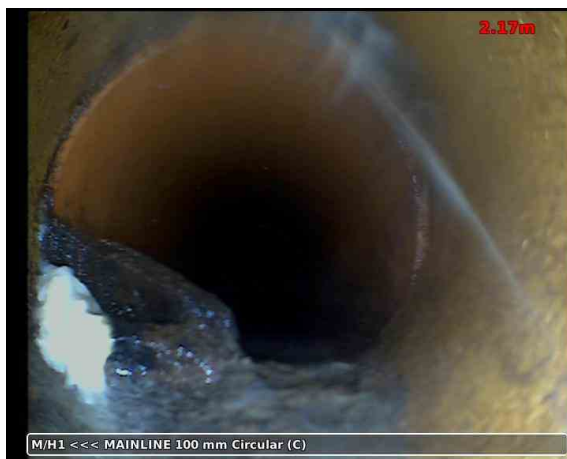
20211118-121526-snap0002.jpg, 00:00:49, 2.17 m Settled deposits, hard or compacted at joint, 35% cross-sectional area loss
