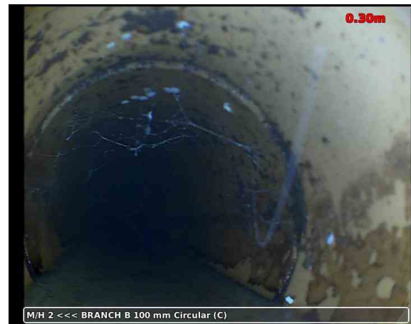
20211118-122550-snap0001.jpg, 00:00:12, 0.30 m Line deviates left
