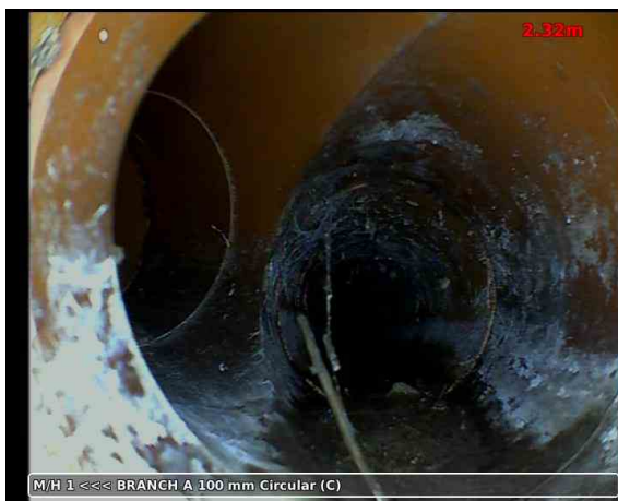
20211118-111324-snap0002.jpg, 00:00:31, 2.32 m Junction at 9 o'clock, 100mm dia
